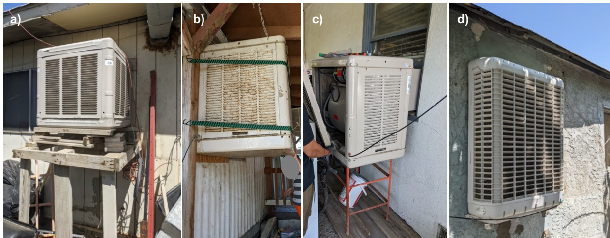
141 142 Figure 1. Sample of EC units observed in the study location during the pilot study: a) horizontal-flow unit 143 installed on a platform, b) horizontal-flow unit suspended by bungee straps, c) through-the-window unit on 144 stand with cover removed, and d) narrow dimension through-the-wall unit.
