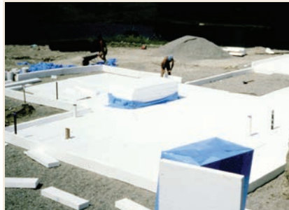
PHOTO 8 Foam Formwork. Float a concrete slab on top of a bunch of foam using the foam as the “formwork” for the slab and leave it in place.
