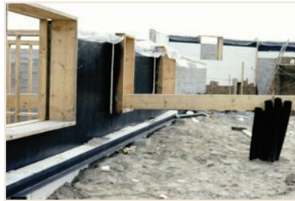
PHOTO 6 Earth Tubes. Note the plastic drain pipes sticking out of the ground. Each pipe was 50 feet in length and connected to the intake side of a heat recovery ventilator.
