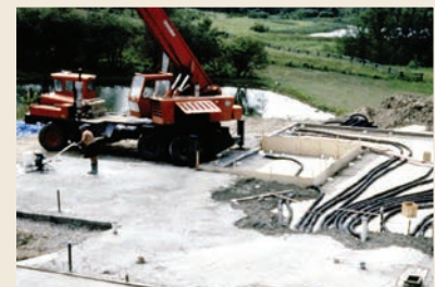
PHOTO 9 (TOP) Ductwork in the Slab. Long coiled plastic drainage pipe was used for the in slab ductwork. Note the fiberglass reinforced polymer modified cement “gluing” the foam formwork together.
